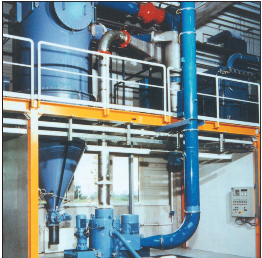
This turnkey system for manufacturing powder coatings uses a Mikro-ACM® air classifying mill model 40. The system is designed to safely contain dust deflagration by means of pressure rated components and explosion barrier valves.
